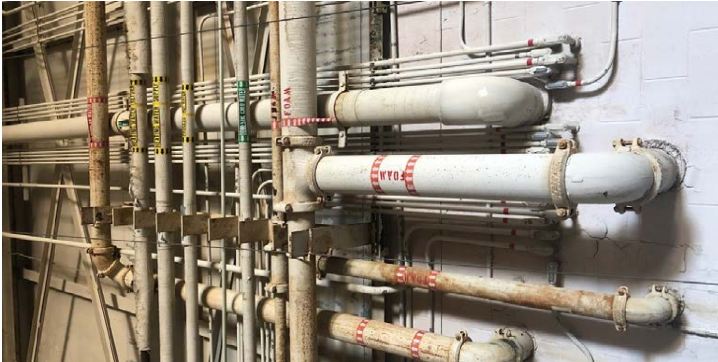
Hensley Field crash structure and monitoring well, 2020
