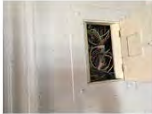
5 Original Electrical Enclosure
