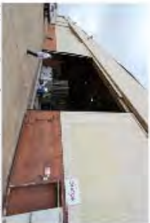
3 Hangar Door System Approx. 24' tall
