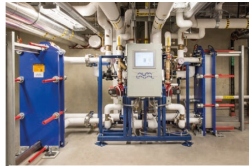
Figure 1: Typical Energy Transfer Station
